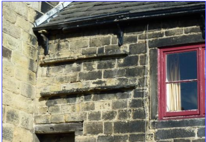
Blocked pigeon holes and alighting ledges at Calverley Old Hall
