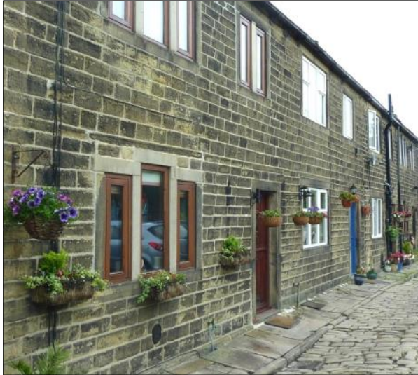
Watershot masonry observed during a YVBSG walk around Wilsden, West Yorkshire
