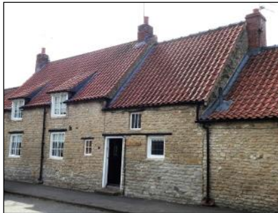
Cruck Cottage, formerly Dixons Cottage (YVBSG 1773). Had at least three pairs of crucks (dendro date of 1512), probably with earthen walls on a high stone plinth and with a thatched roof. Main housebody floored over in late C17 and fine hooded fireplace assembly inserted. In C18 or C19, part of byre was converted to a kitchen which remained open to the roof, while the rest of the byre remained in agricultural use for some time.
