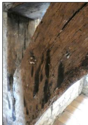
Burn marks on a brace in the Hall
