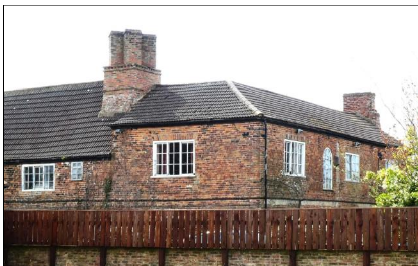
Above and top right: Distinctive chimney stacks at Bagby Hall Farm, Bagby, North Yorkshire – one of the Group's early reports dating from 1970 and comprising only a short description with two photographs (YVBSG 0004). Should our future activities involve updating earlier reports?
